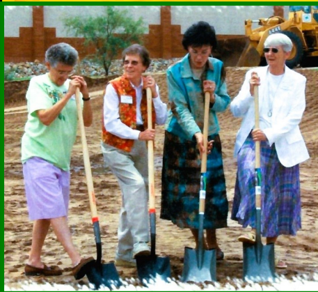
Groundbreaking for the West Wing Pat Byers, Ann Slagter, Jean Davis, Artie Collins August 6, 2007
